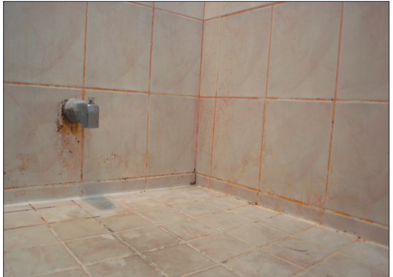
Water that has wicked into building materials behind a tile wall can leach out into the grout and even into stone tiles to cause serious stain issues.
