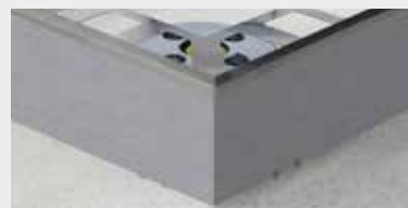
F5. Wedge the cut tile between the BSJ profile and the SUPACLPB clip.
