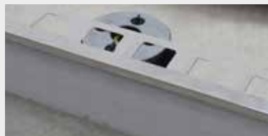
E5. Wedge the cut tile between the BSJ profile and the SUPACLPB clip.
