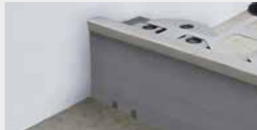
D5. Wedge the cut tile between the BSJ profile and the SUPACLPB clip.
