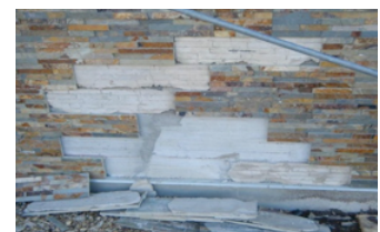
Delamination of Stone
