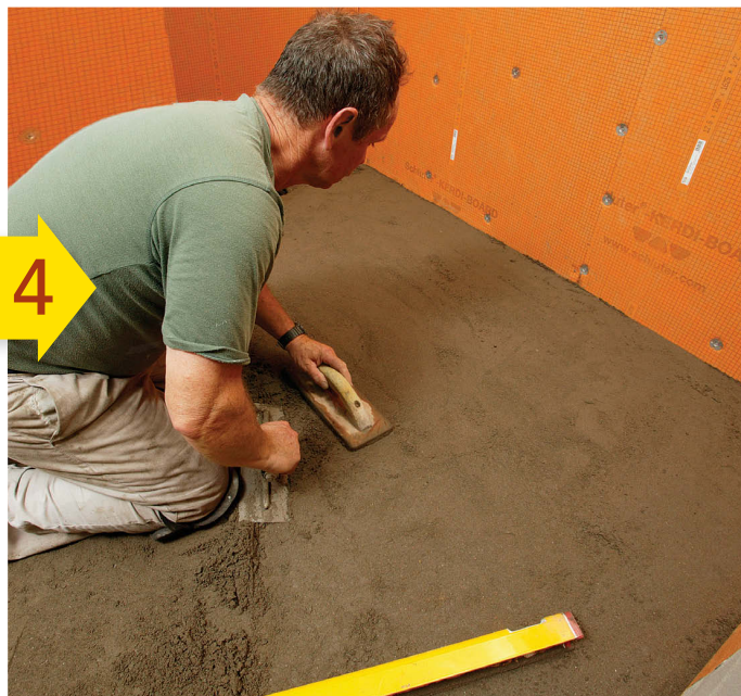
Smooth transitions. Once the pitch is established, use a wooden float to grade the transition from the level floor to the shower along the side.
