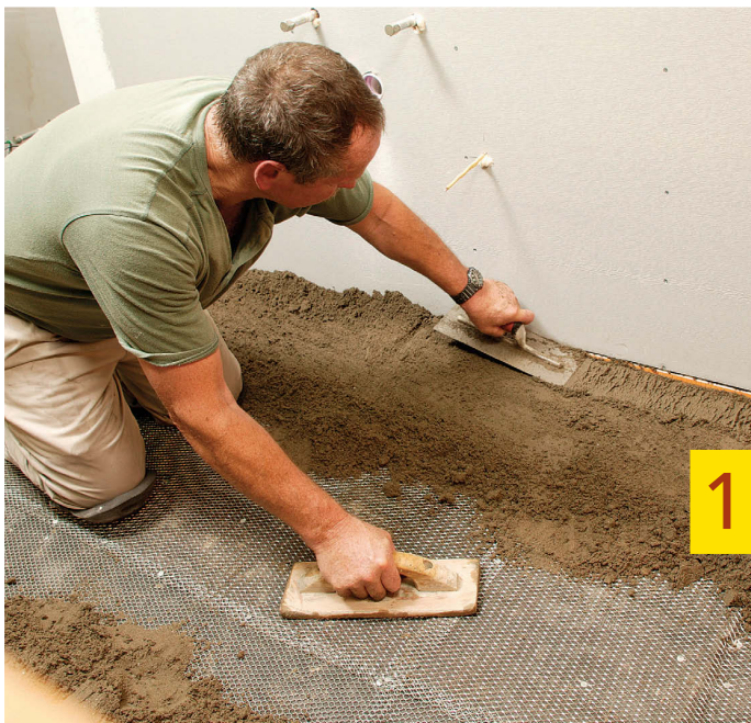
Pack and level. On the level part of the floor, use a steel trowel to pack down the loose mortar so that it forms a level perimeter about 1 in. thick around the room.
