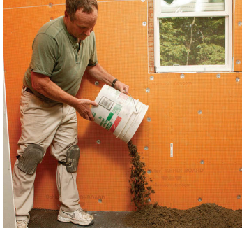
Dump the mortar. Use a 5-gal. pail to distribute piles of mixed mortar evenly around the perimeter.
