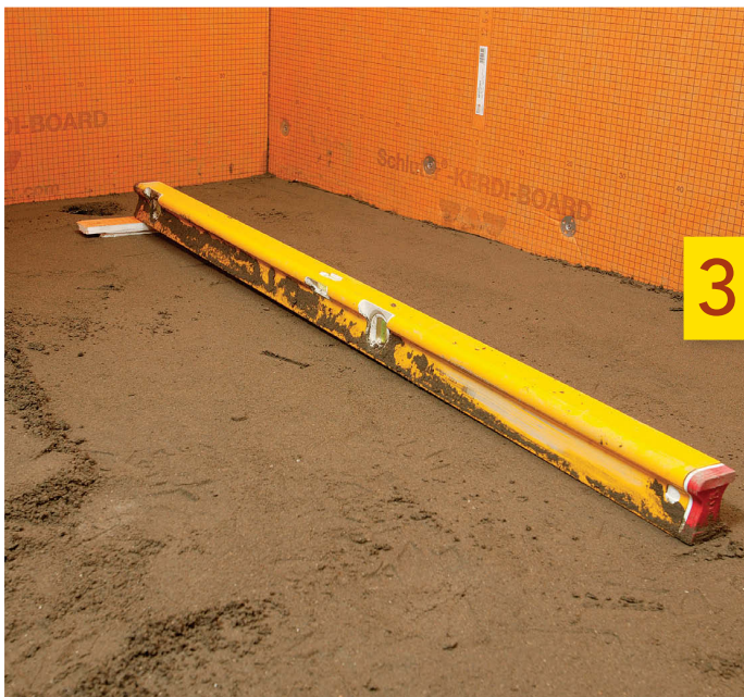
Create the pitch. In the shower area, extend the level floor grade to the high end, then create a single slope to the drain. The total difference in grade should be about \frac{3}{4} in. for a 3-ft.-long shower like this.
