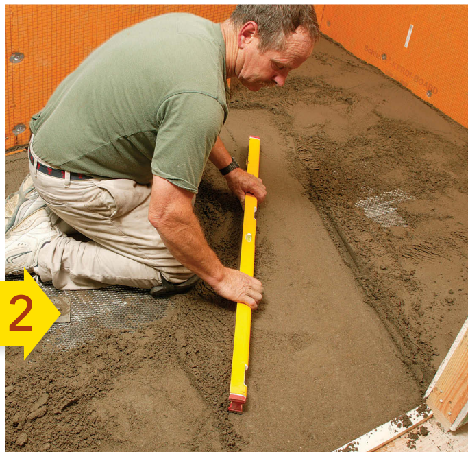
Fill and screed. Dump more mortar in the middle of the floor, and pack it down. Use a level as a screed, resting one end on the perimeter as a reference for the floor's center.
