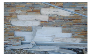
Delamination of Stone
