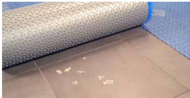
Existing cracked tile
