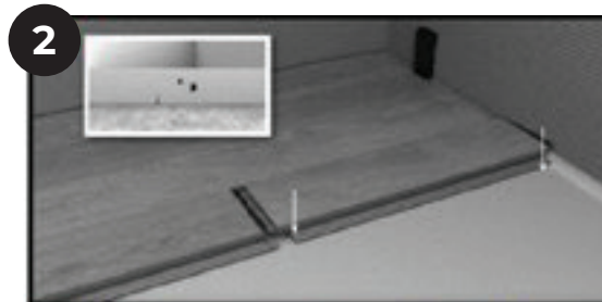
STEP 2: Slide plank toward end of previously installed plank until the tongue just touches the groove.
